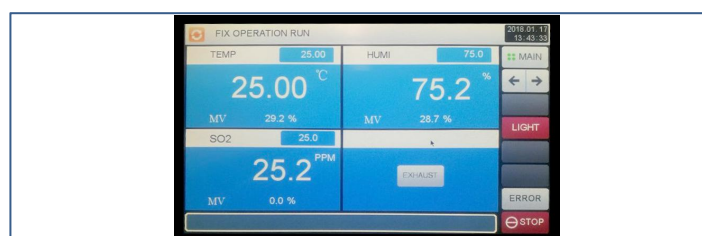
SO2 Control system
